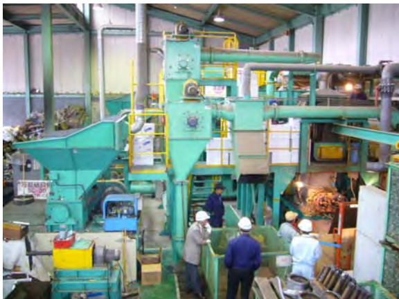
Figure 3.6: Smaller RPF production facility (150 kg/h capacity)
